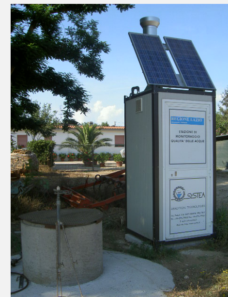
Self powered ground water station
